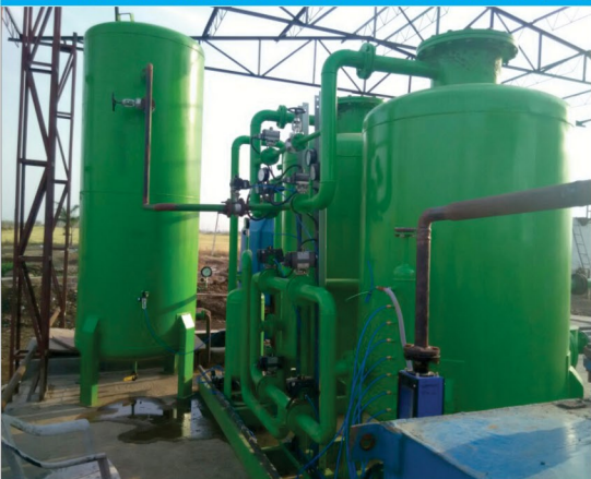
VPSA Biogas Purification Plant
