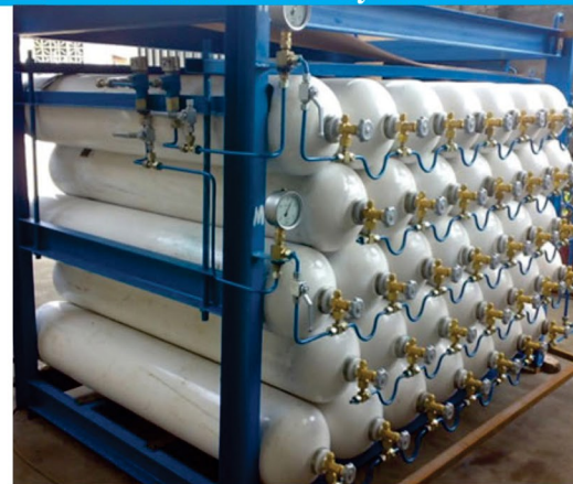
Cascaded CNG Cylinders
